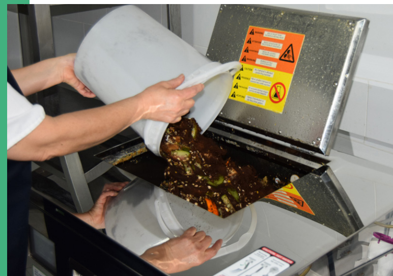
Biogas digester installed at ILUNION Hotels
